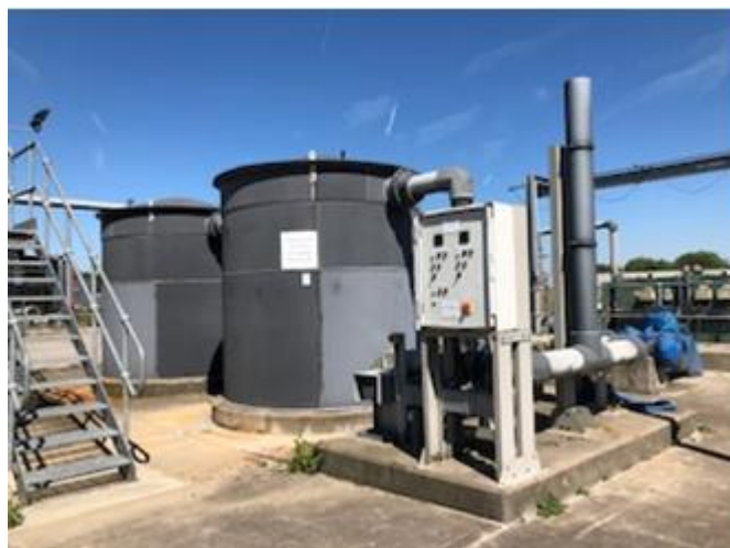
Figure 4: Peacemaker System in series at sludge import area
