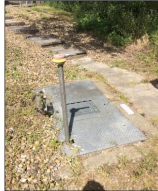
Figure 4: Condensate trap, near flare stack.
