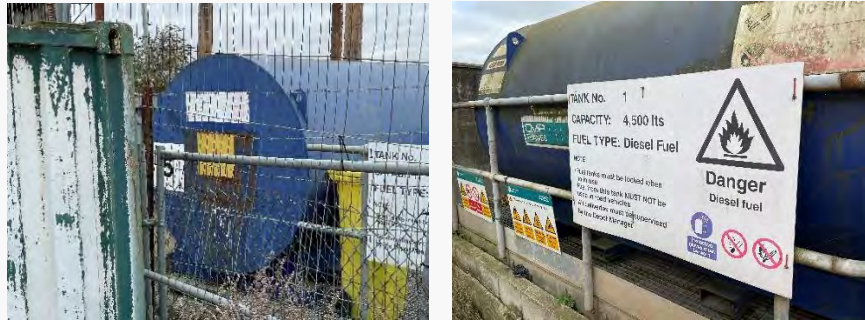
Plate 2.1 Above Ground Diesel Tank (Source S1)
