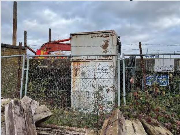
Plate 2.6 Electrical Transformer/Switch gear (Source S4)
