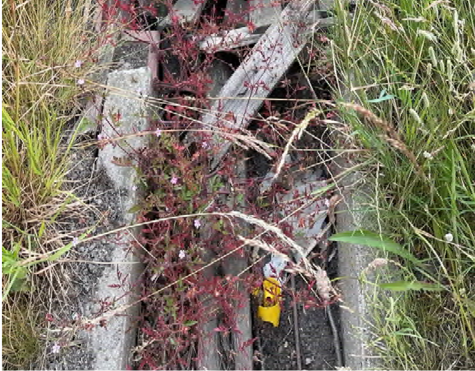
Figure 2.3 Blocked existing drainage channel
