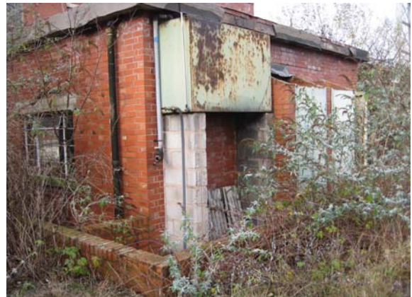
Photograph 4. Above Ground tank near to transformer compound
