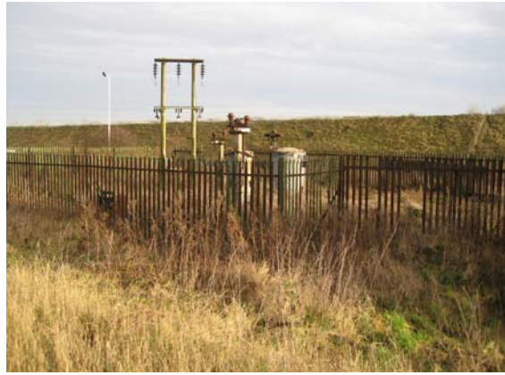
Photograph 8. Sub station (council owned land) south of the former power station
