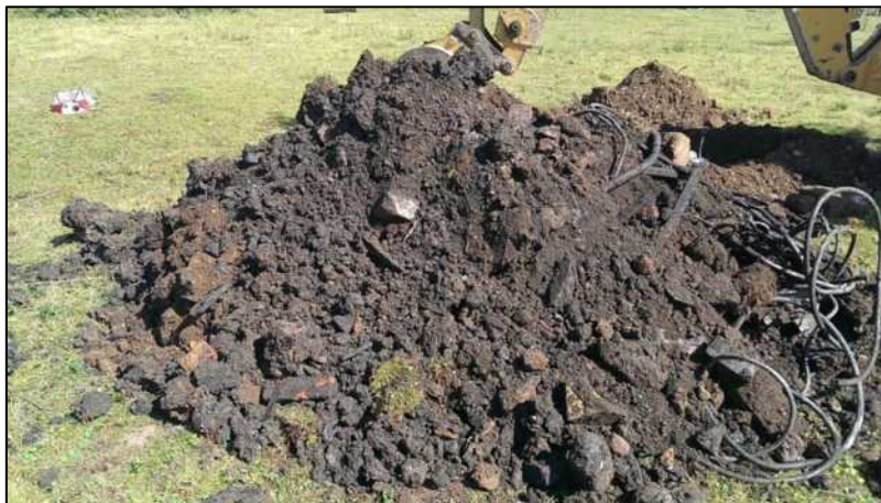
Photograph 22: TP6 - Arisings from between 0.9m and 3.5m together with electrical cables.
