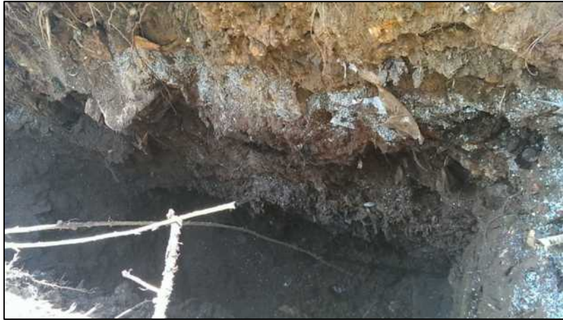
Photograph 4: TP2 - Shattered plastic layer at 0.4m at the change between the orangey brown sand and the organic blackish clay containing concrete, rubber, bricks and other material. The black clay had a hydrocarbon odour.
