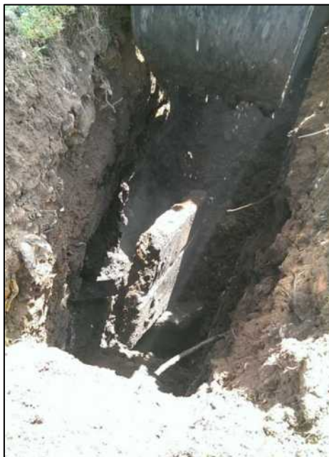
Photograph 24: TP6 - One of three large concrete slabs measuring between 500mm and 800mm in length.
