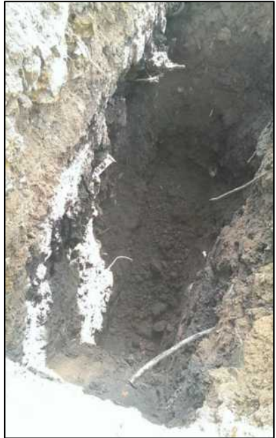
Photograph 25: TP6 after collapse of the blackish sand and rubble between 0.9m and 3.5m.
