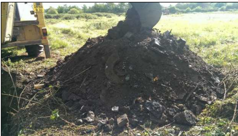
Photograph 9: TP3 - Blackish brown sand arisings containing concrete, plastic, metal, bricks and fabric. Black sand had a hydrocarbon odour.
