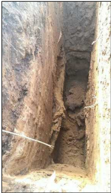
Photograph 3: TP1 - Collapse of the silty sand at 2.4m
