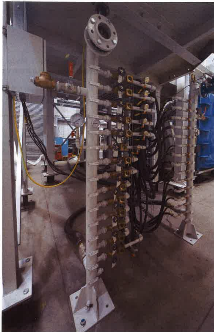
Typical Consarc Supply and Return Water Manifolds
