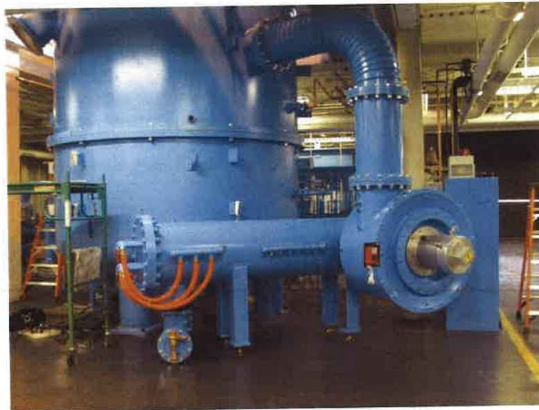
Typical Heat Exchanger and Gas Fan
