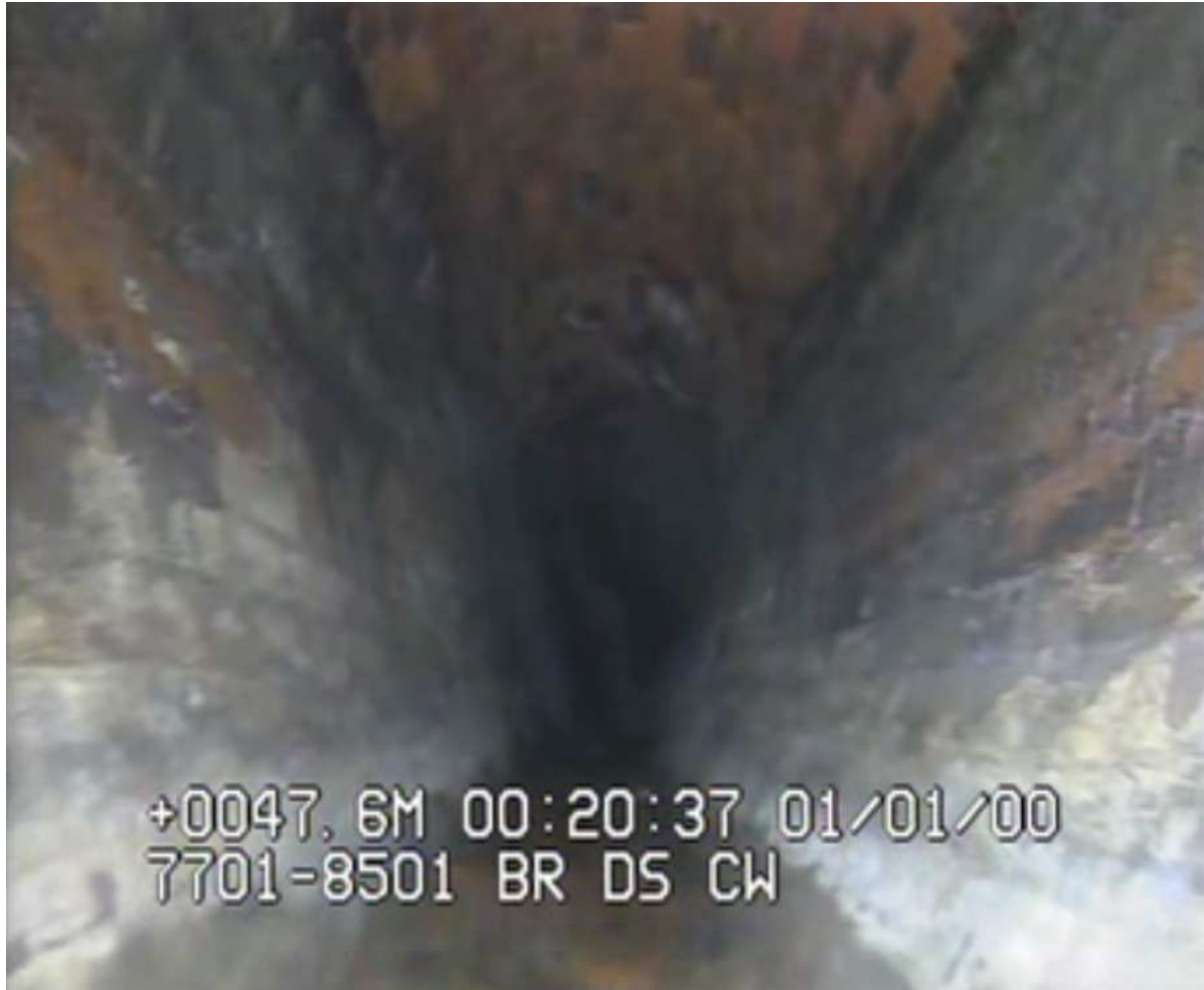
Shallow depth of water downstream of manhole 7701
