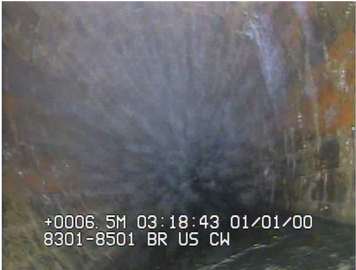
Silt and standing water downstream of manhole 8501
