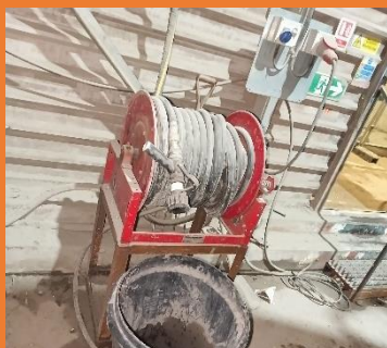
Main Fire Fighting Point
