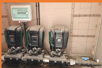
Auxiliary Fire Fighting Point
