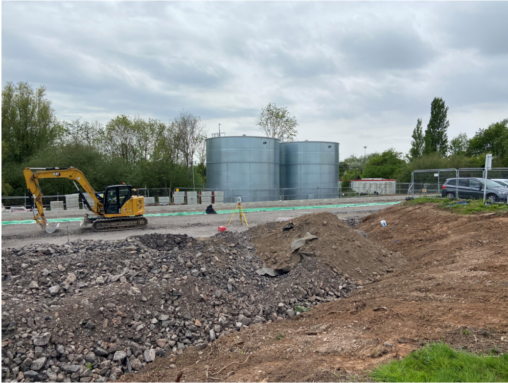
View NE of development works W of existing building; Water tanks in the background.
