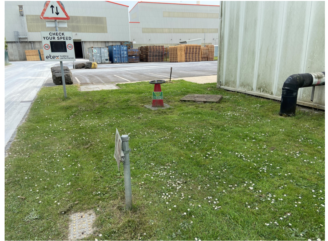
Pollution Control Valve
