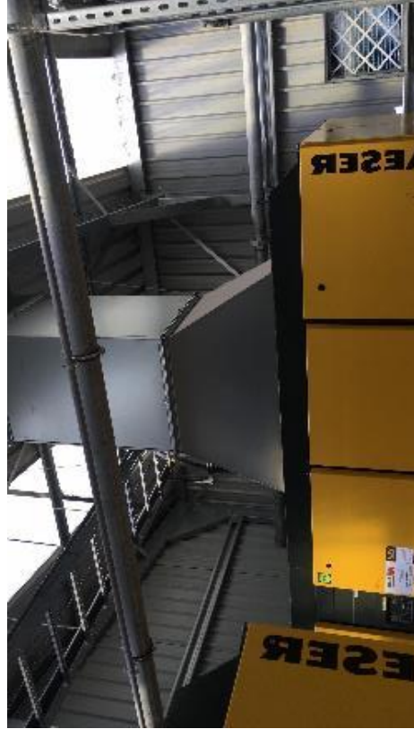
Additional compressor room
