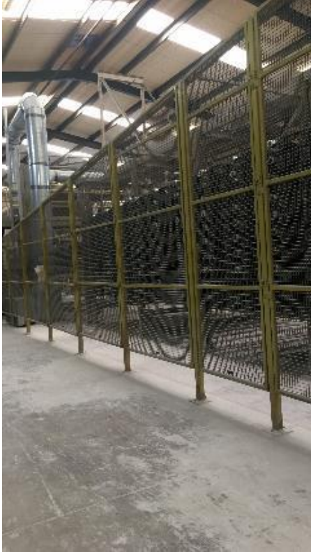
Alongside oven entrance
