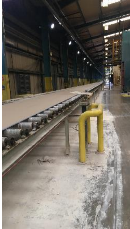
Wetside to Dryside conveyor/Oven system
