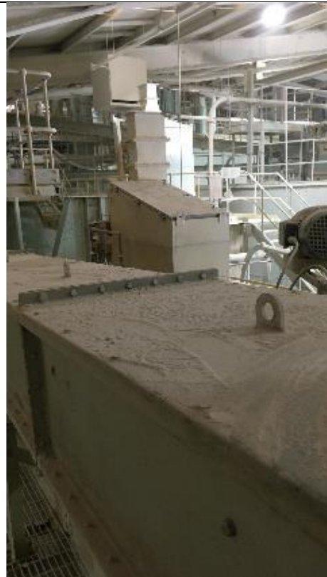
Conveyor system above mixer
