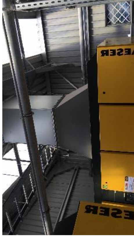
Additional compressor room
