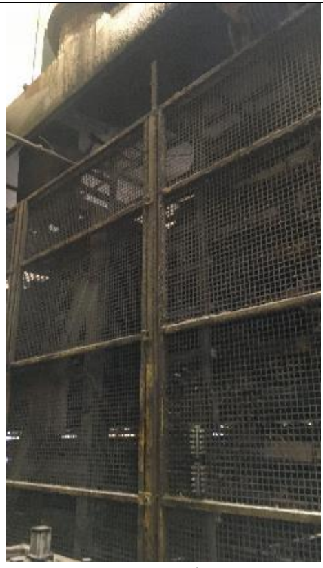
Conveyors near start of ovens
