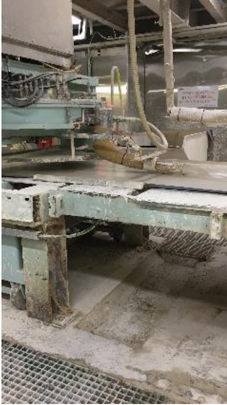
Mixer outlet area
