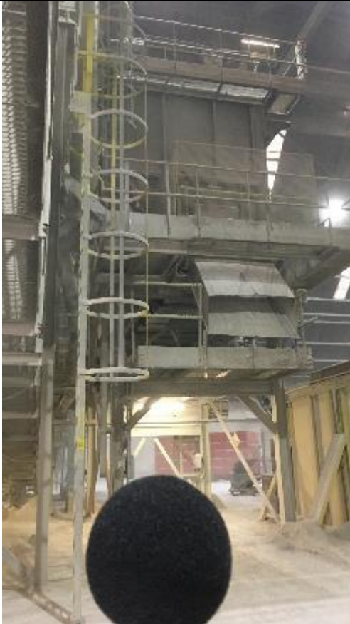
Conveyor centre of gypsum storage
