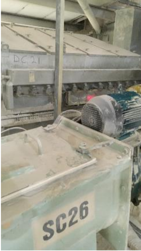
Silo above mixer
