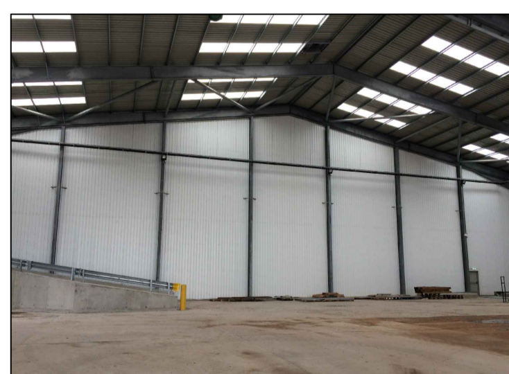
Acoustic Cladding In Storage Building
