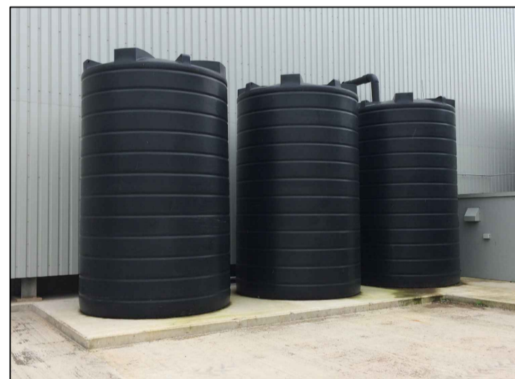
Harvested Rain Water Tanks
