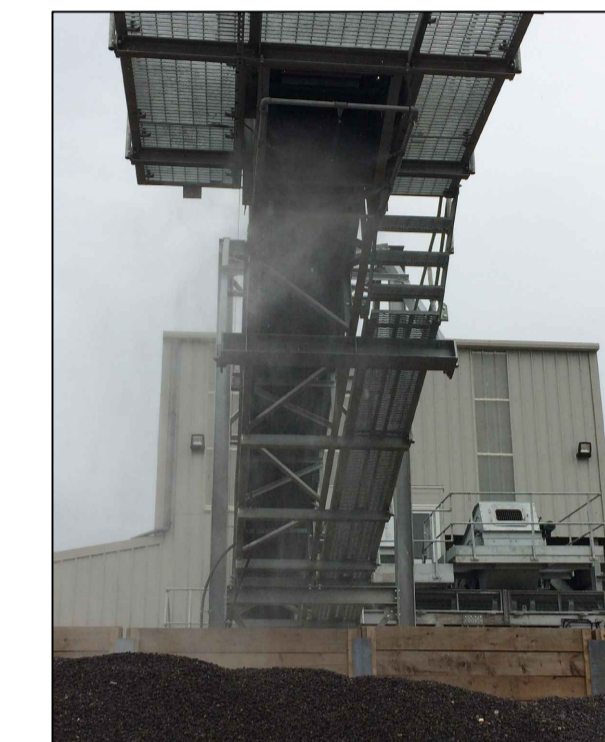
Conveyor Head Halo Spray
