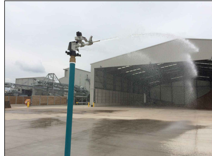
Yard Dust Suppression Units
