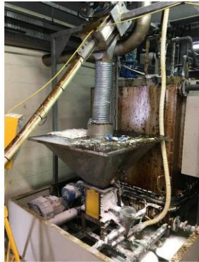
Figure 3: Polyelectrolyte conveyor and dosing station
