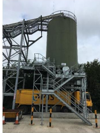
Figure 4: Post-digestion sludge cake storage silo
