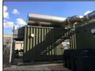
Figure 20: CHP plant, Finning Power Systems.
