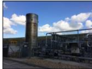
Figure 21: Flare stack compound.
