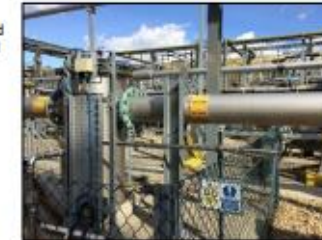
Figure 23: Condensate receiver, flare stack.
