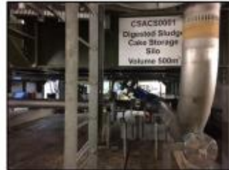
Figure 13: Equipment below silo.
