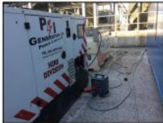
Figure 24: Temporary generator & diesel tank.
