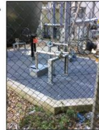
Figure 19: Condensate trap, gas holder compound.
