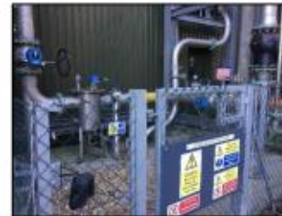
Figure 22: Condensate receiver, dryer building.
