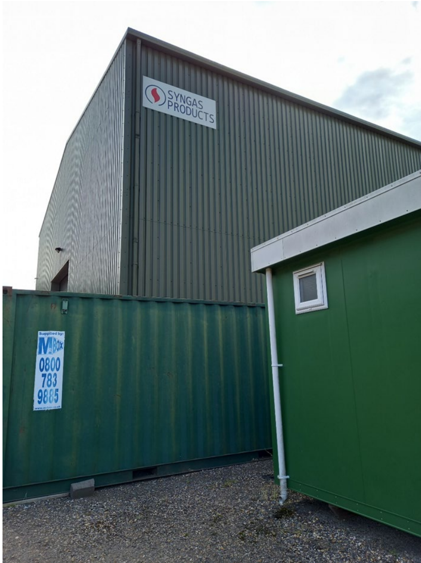
Image EDP A3.1: External construction of the main structure (B1) and a portacabin
