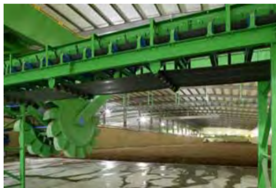
The beam which holds the compost turning wheel in place has broken
