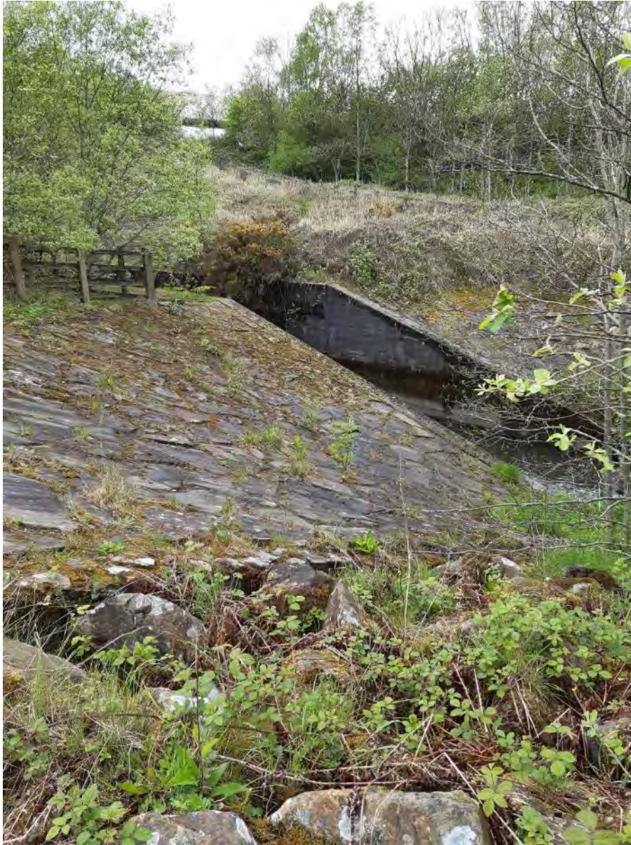
Plate 7, Davy Field Brook entering culvert under motorway to north of the site.
