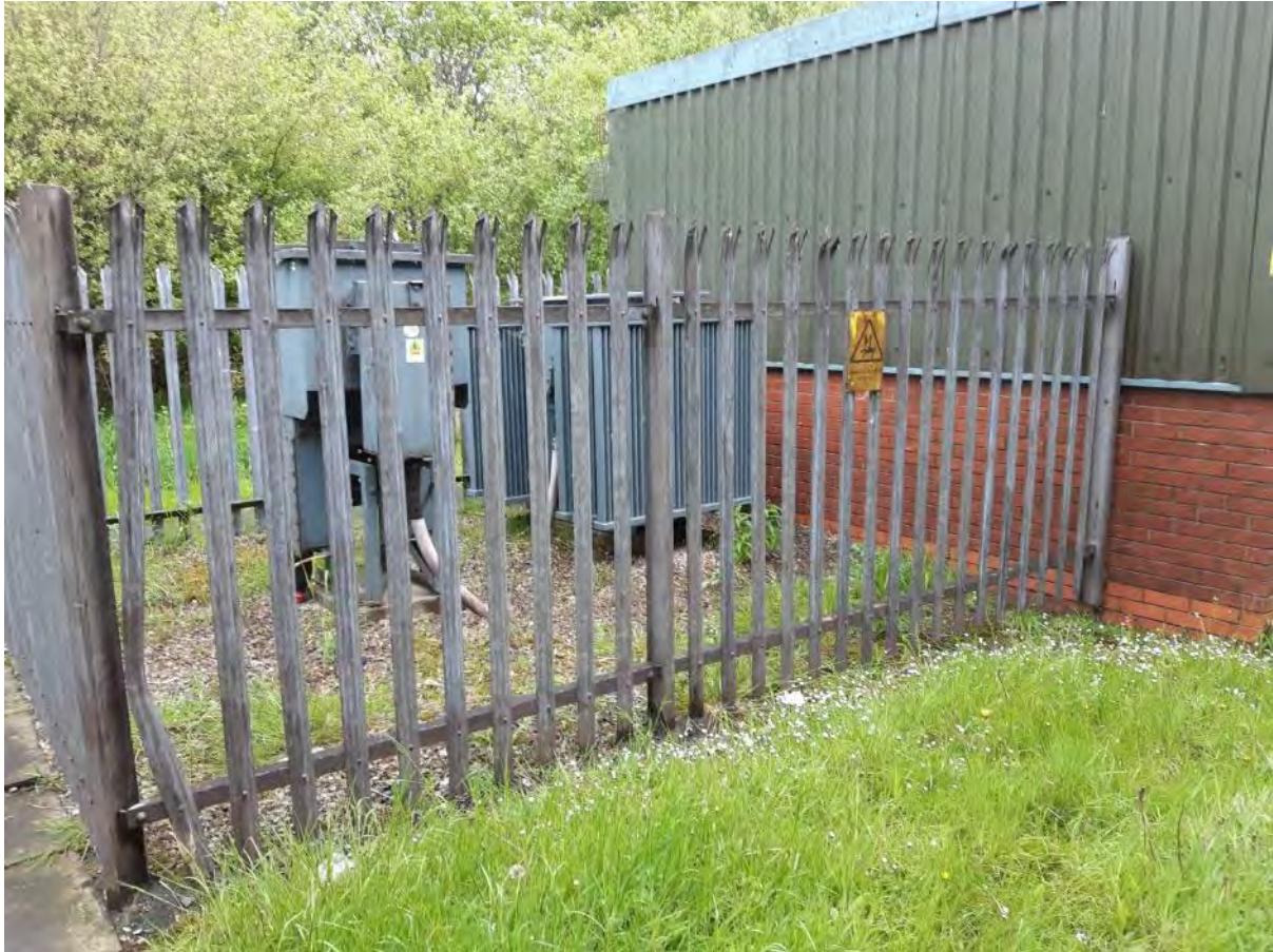
Plate 10, Onsite substation to north of the ink building
