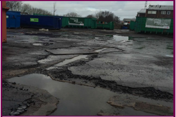
Photo 14: Hardstanding in poor condition
