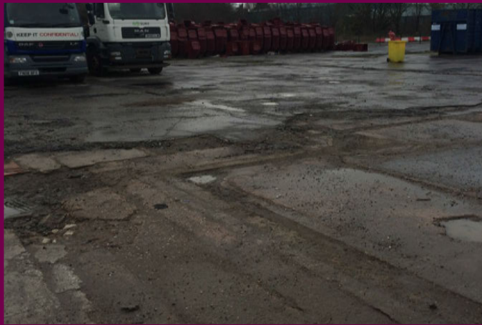
Photo 15: Hardstanding in poor condition
