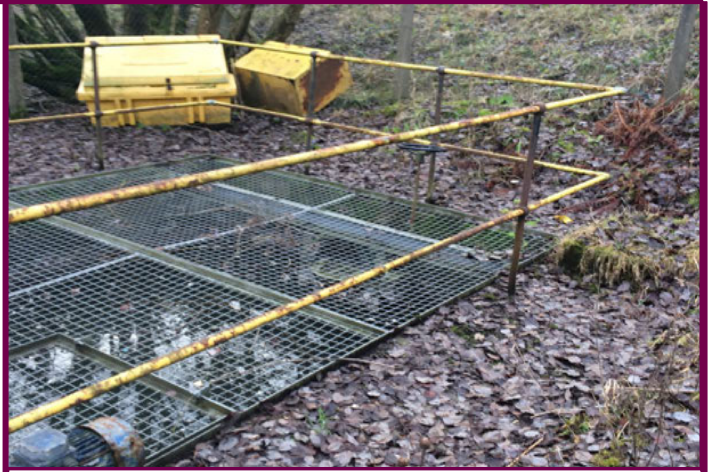
Photo 20: Large interceptor tank in north of site
