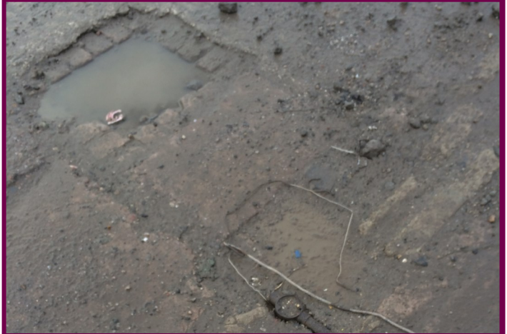
Photo 16: Standing water in voids
