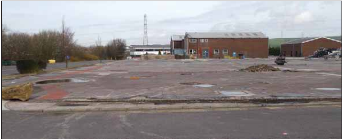
Figure 6 – Photo looking north from SW corner of proposed warehouse building. Photo shows existing concrete slab.
