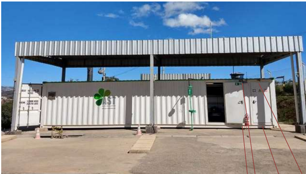
Figure 1 – Three stage RO System, 200 m3/d, Brazil, Maceio.
