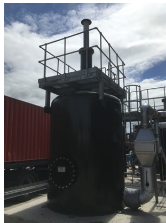
Figure 11: Biomethane GAC odour control unit.
