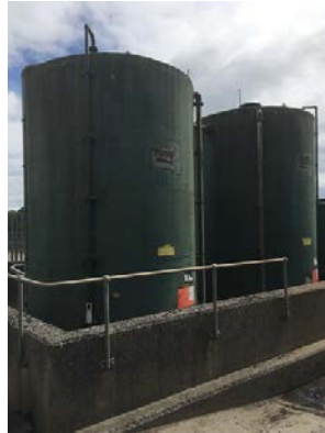
Figure 10: Ferric sulphate tanks at Trowbridge WRC.
