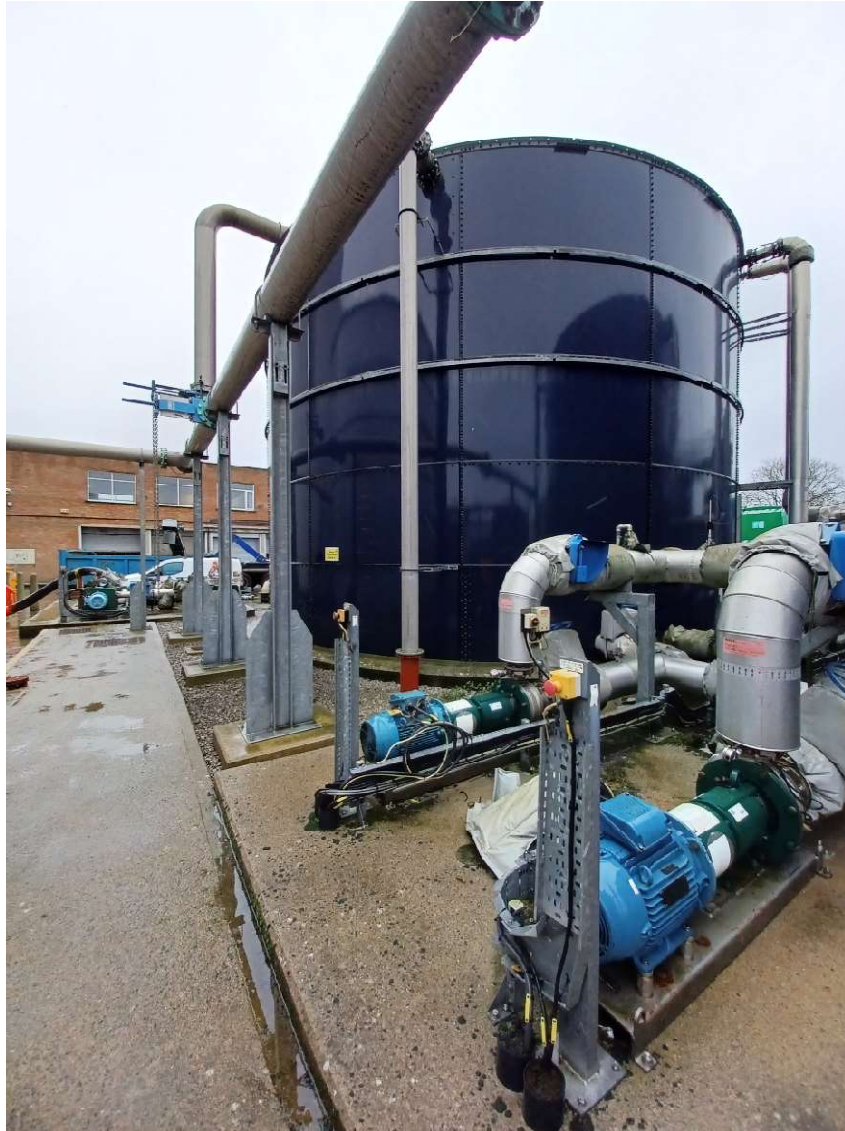
Figure 8.13 Secondary Digester Tanks
