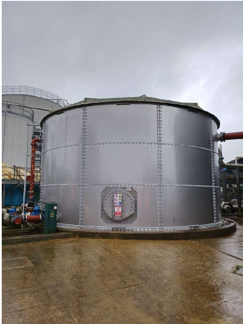
Figure 8.1 Sludge Reception Tank
