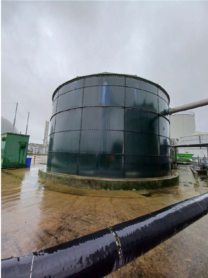
Figure 8.3 Pre-Thickened Storage Tank 1
