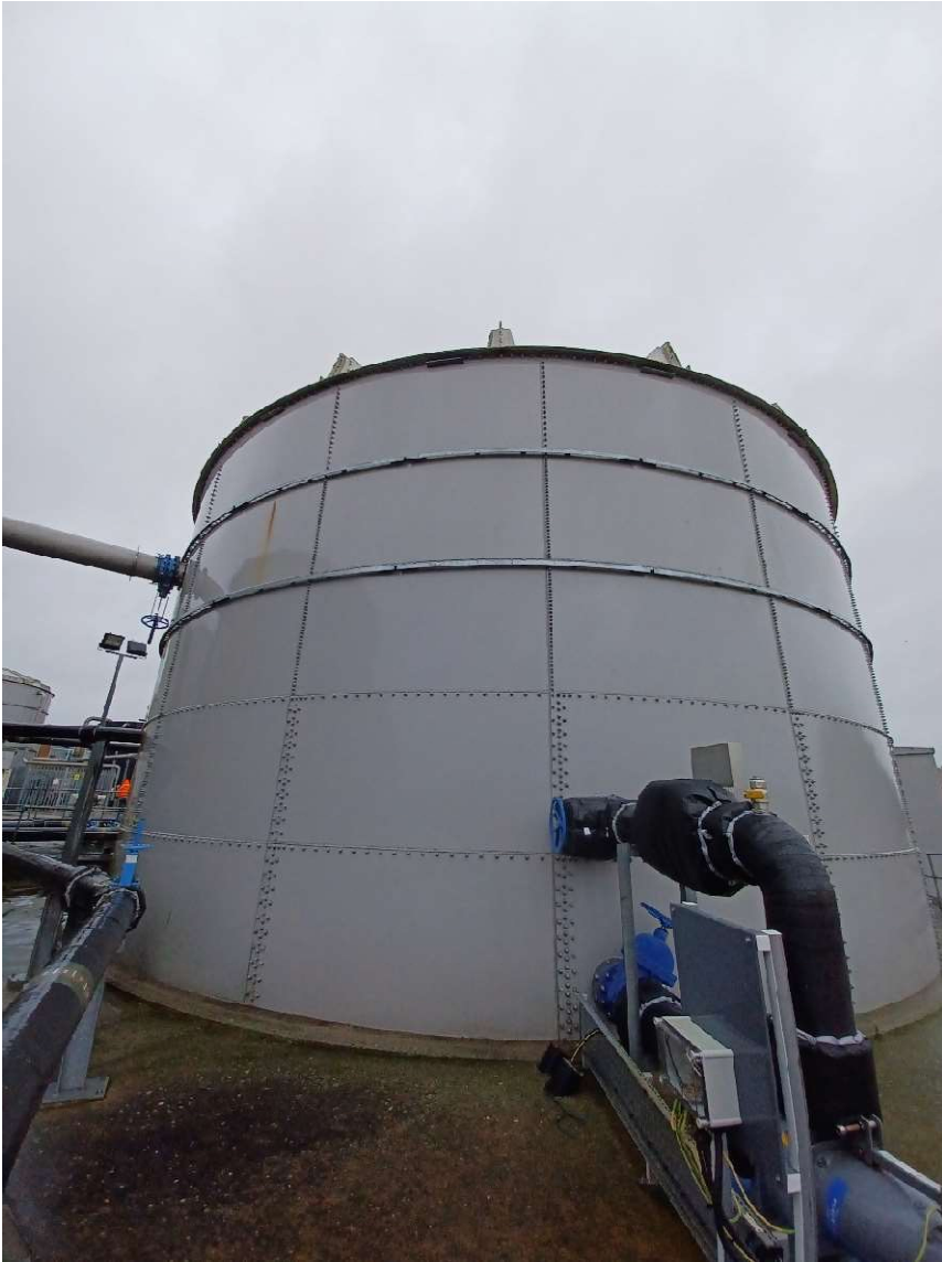
Figure 8.5 Pre-Thickened Storage Tank 2
