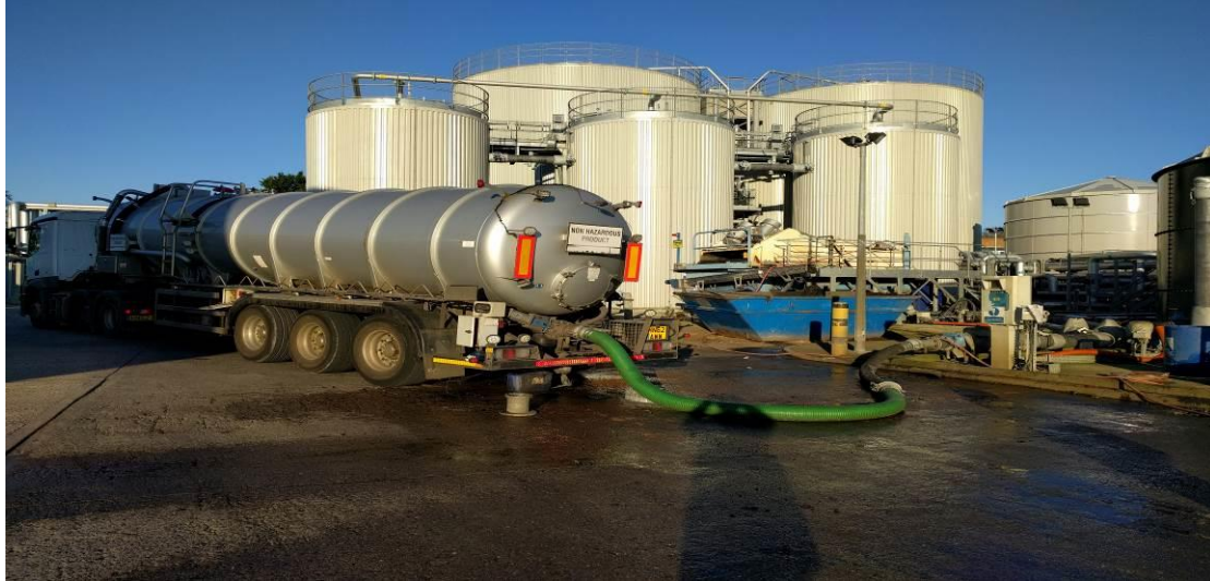
Sludge Import discharge point
