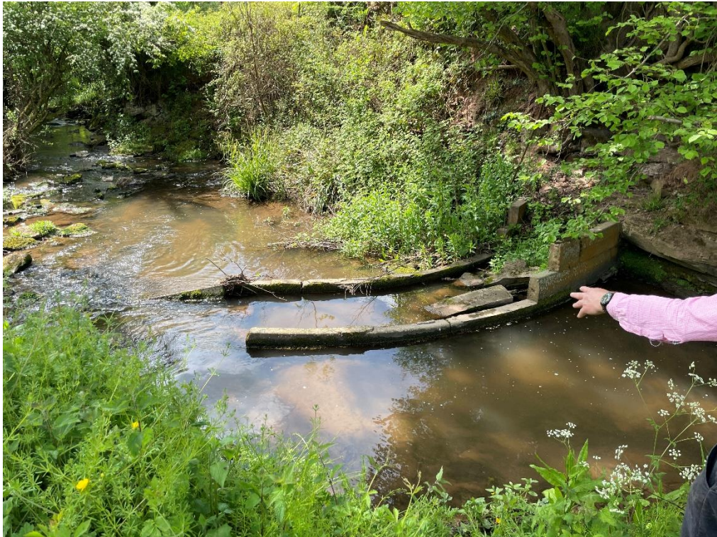
Figure 2. The failed weir.
