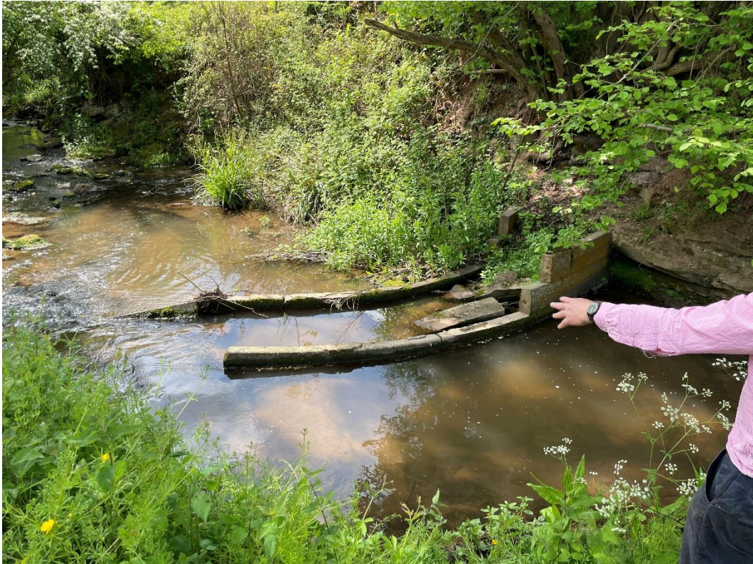
Figure 1 Image displaying the failed weir on the Hollands Mill site.
