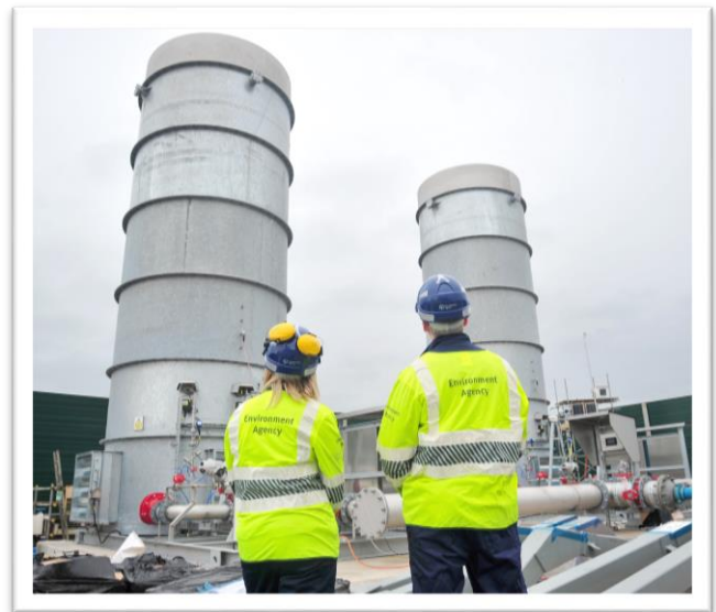
The two flares at the Preston New Road site
