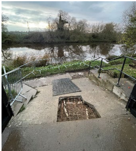
Figure 1 – Site investigation works to check the sheet piles underneath the flood wall. This has been re-instated.
