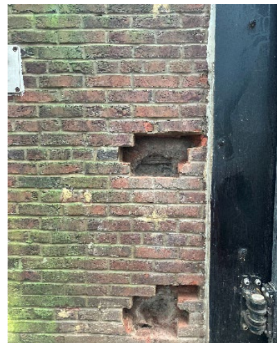
Figure 2 – Investigation of the re-inforcement within the flood wall. This has been re-instated
