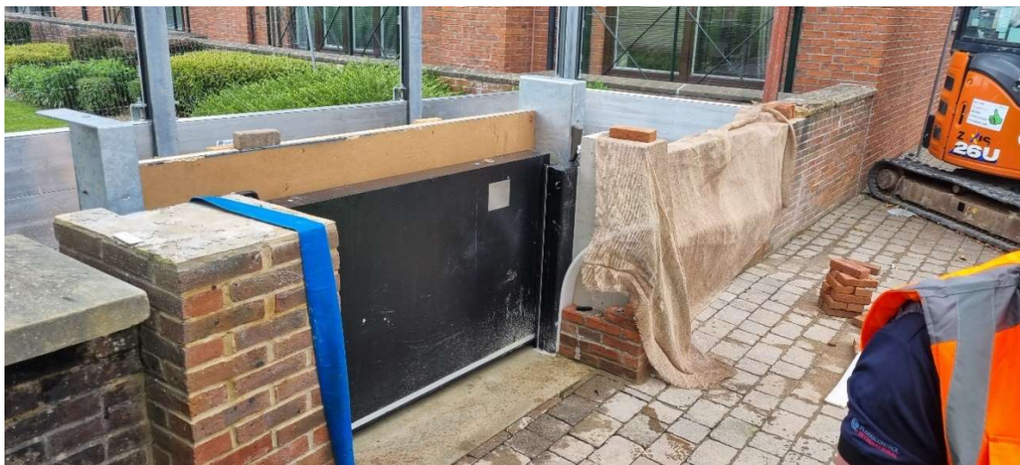
Figure 3. Gate 31 following installation. With preparation on going for the water test. Also seen are the temporary Flood barriers installed to continuously protect Yarm when the old flood gate is removed.
