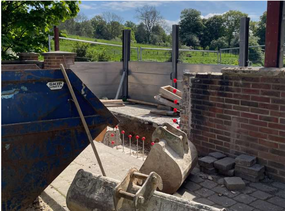
Figure 2. Gate 31 prior to installation, showing the temporary flood defence required to allow the work to proceed and maintain the flood protection level of Yarm.
