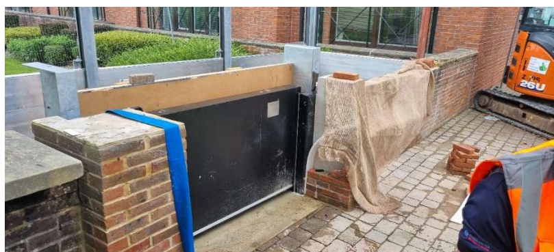
Figure 2. Gate 31 following installation. With preparation ongoing for the water test. Also seen are the temporary Flood barriers installed to protect Yarm when the old flood gate was removed.
