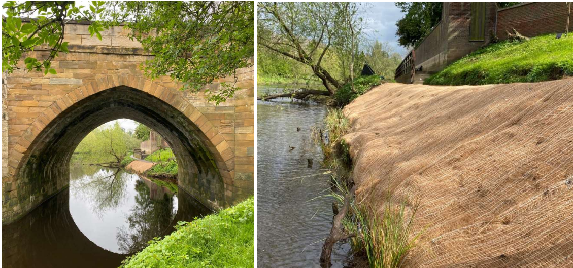
Figure 6&7. Environmental Enhancements - Installation of coir to protect the bank surface or bank toe.
