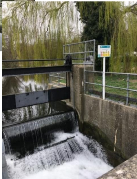
Image right: Cogglesford Sluice tilting gate one of many moveable structures on the Slea. It is used to retain water levels within the River Slea and allows water to pass when water levels are high to reduce flood risk.
