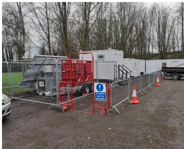
A Hydrogen Fuel Cell used to power the site
