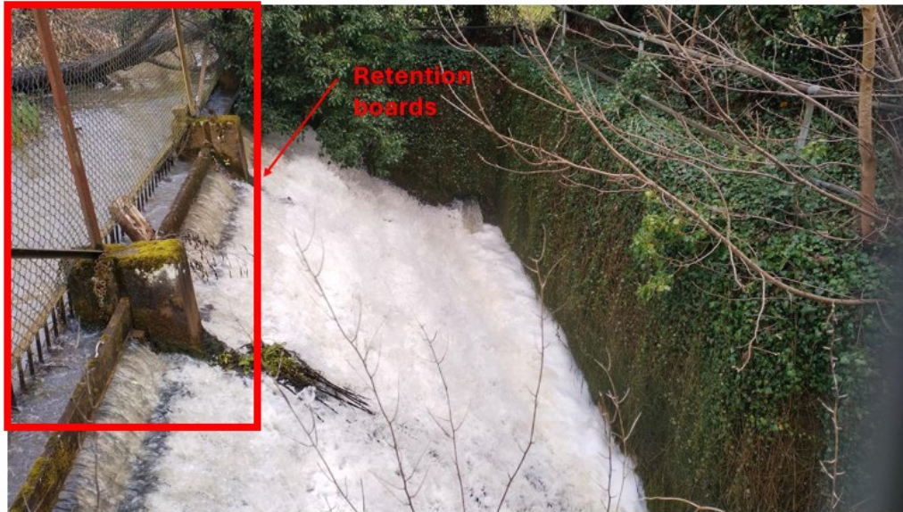
Image showing flood weir and where retention boards are currently inserted (red box) during periods of low flow.
