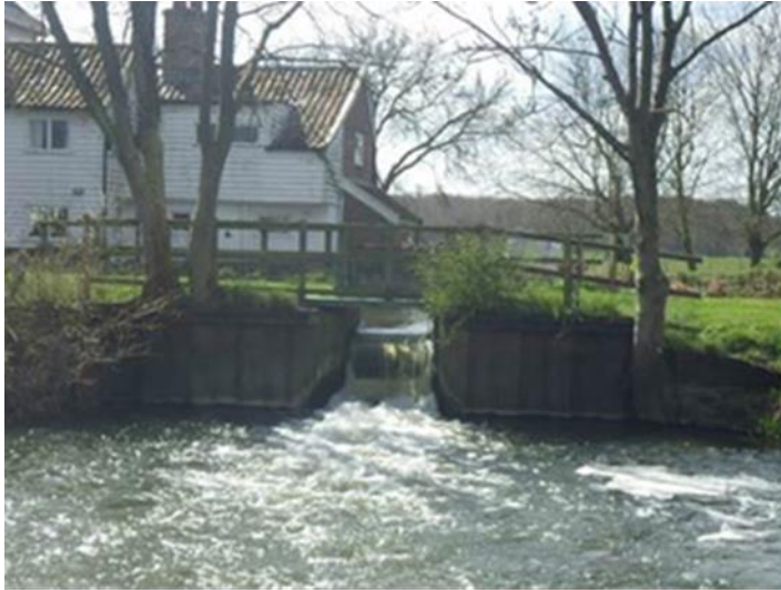
Photograph 1: Environment Agency maintained mill sluice at Wortwell Mill
