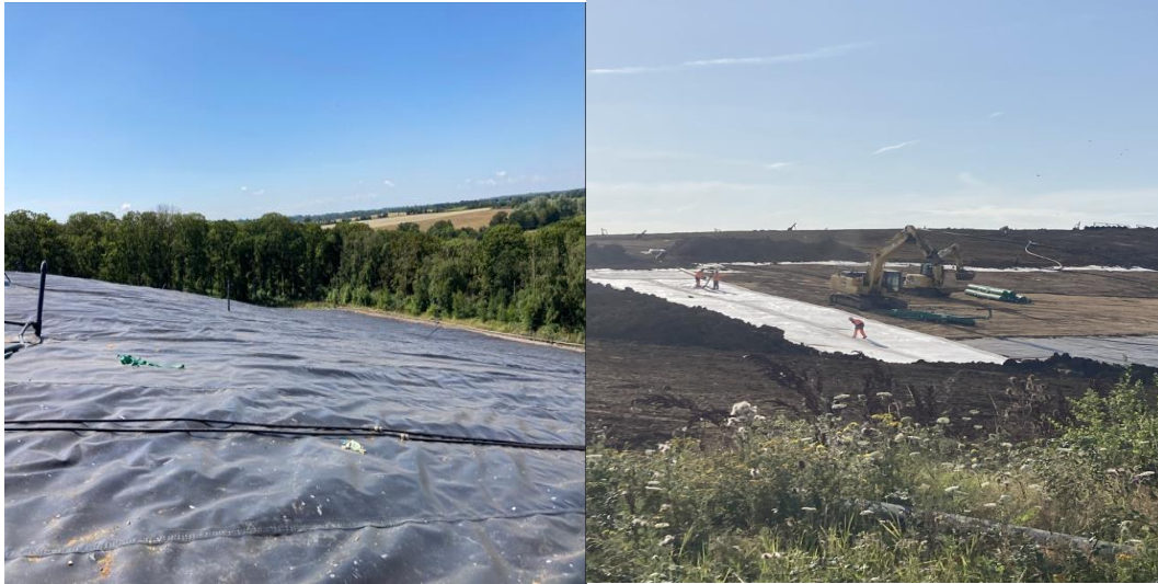
Left - temporary plastic cap+ gas Cell 9-10 western flank. Right – permanent capping being installed
