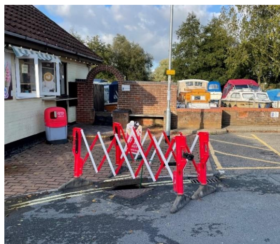
Figure 3 - Surface water penstock on Fen Lane
